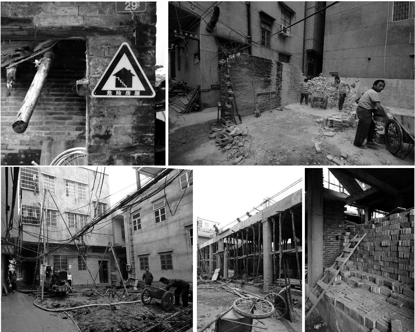
Figure 2: The process of disassembling and salvaging brick from older buildings, pouring new foundations for new, multistory concrete frame structures, and the return of bricks to be fitted in as infill plays out across the village on many different sites.
